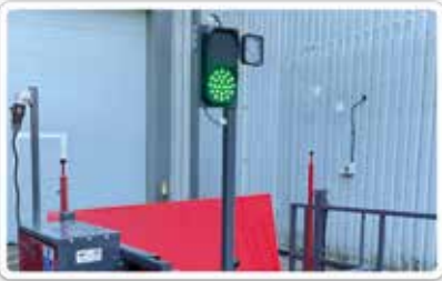
▲ LED Traffic Lights Interlocked to control panel
